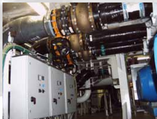
Seawater cooling pump room
