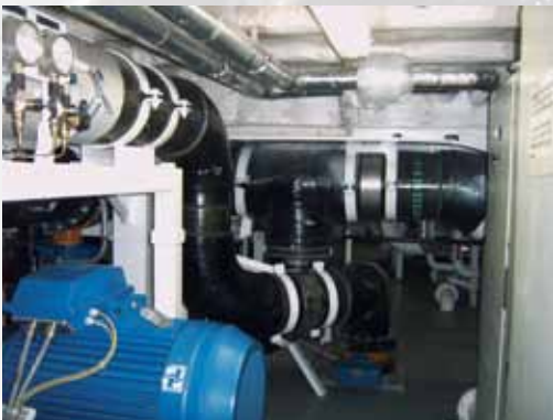
Ballast pump room
