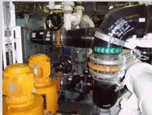
Seawater cooling system
