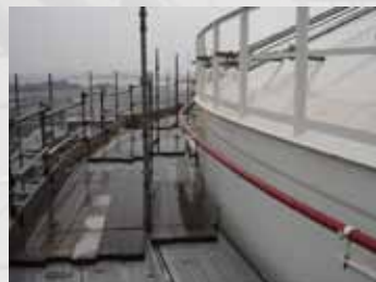
Sprinkler line bent around tank
