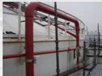
Riser pipe to sprinkler system
